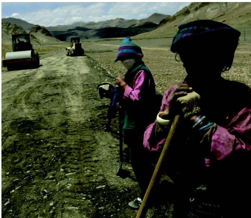
Workers stand on the construction site of the highway to Mount Everest, at Dingri County, Tibet. June 2007
